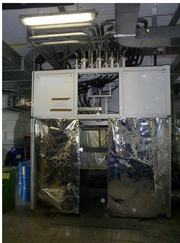
Photo 2: Dosing station for mobile bins with exhaust air extraction and curtain.
