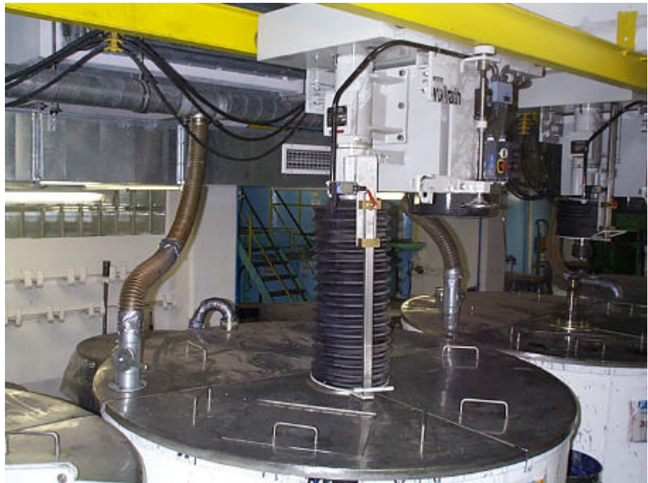
Photo 15: Finish tanks with exhaust air extraction via flexible hose and concertina expansion joint at the agitator shaft.
