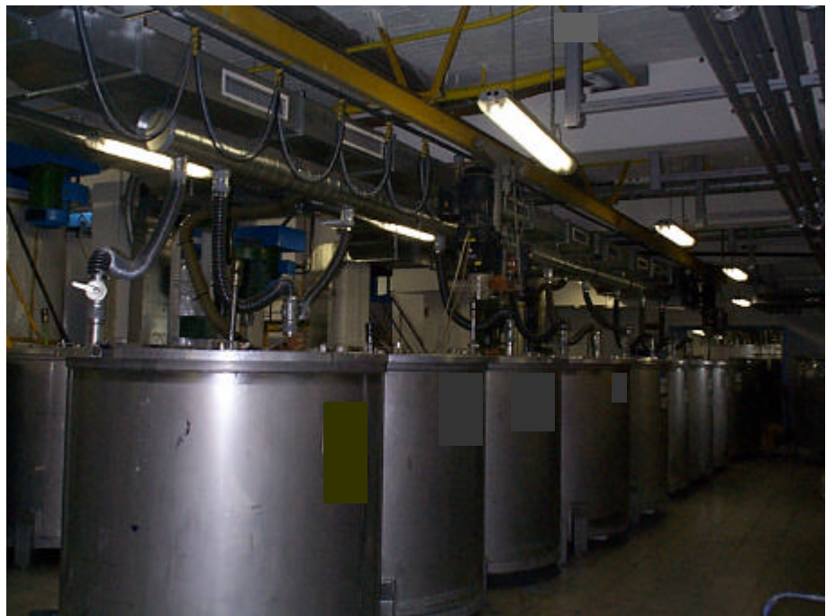
Photo 16: Finish tanks with exhaust air extraction via flexible hose and exhaust air piping system and above the ventilation system for the working environment.
