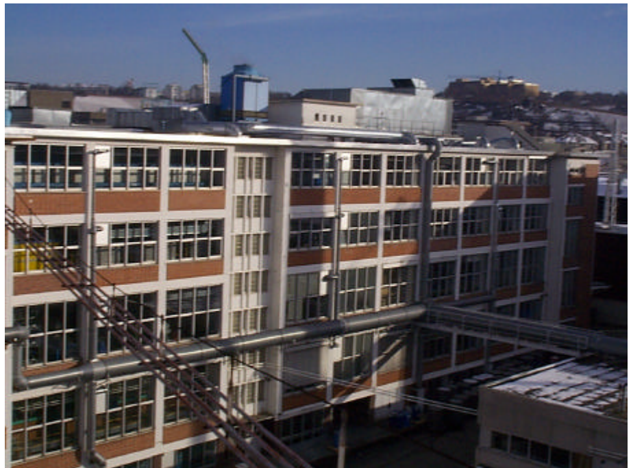
Photo 2: Collecting pipe system for exhaust air from the production building.
