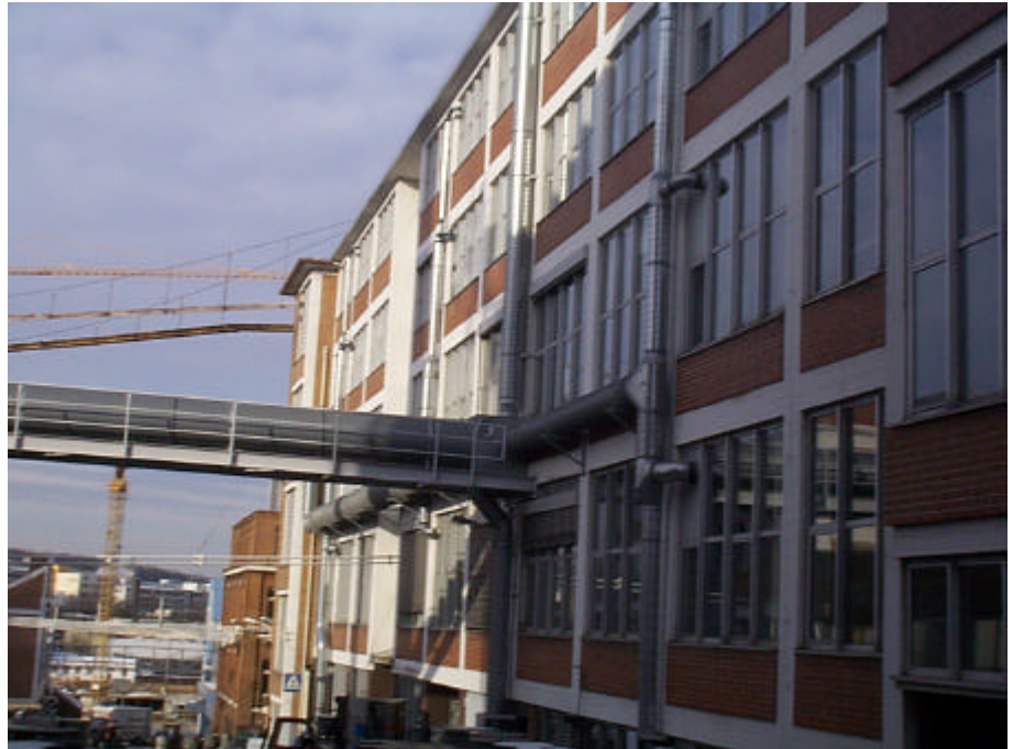
Photo 1: Collecting pipe system for exhaust air from the production building.
