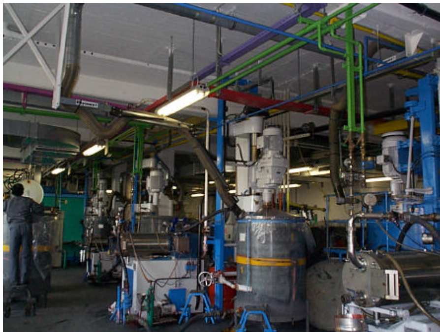
Photo 5: Dissolver with mobile bin and exhaust air extraction by flexible hose during dosing of liquids and dispersing.
