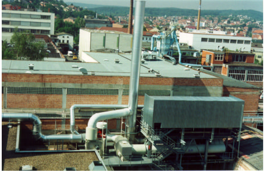
Photo 3: Thermal regenerative combustion plant.
