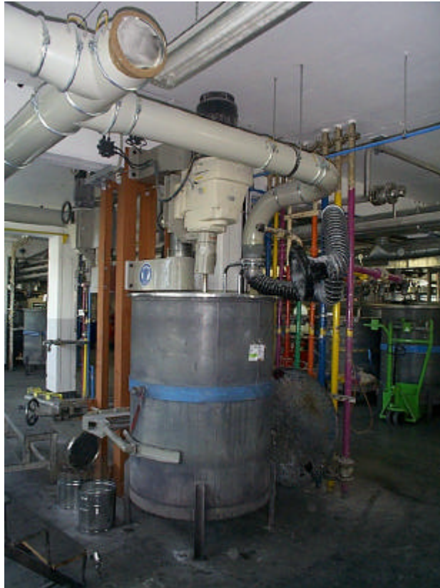
Photo 7: Dissolver with mobile bin and flexible hose with extraction hood.
