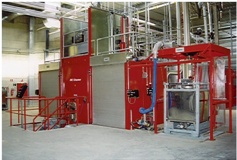
Photo 6: External rinsing station (Riobeer, IBC cleaning plant CW-III-ex 3D).
