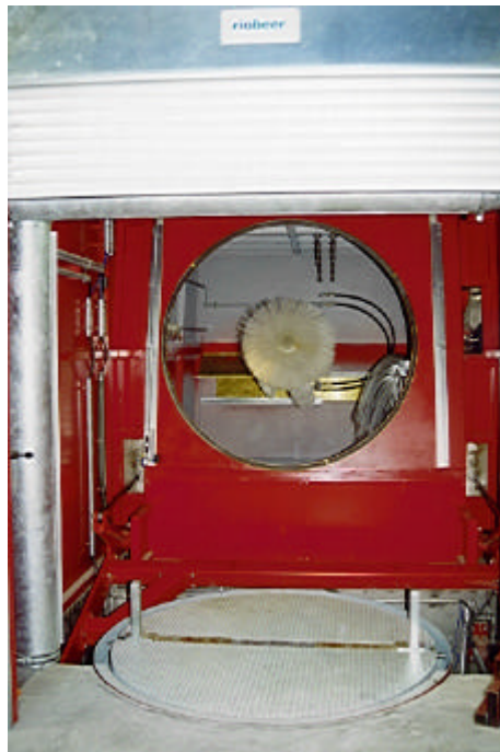
Photo 9: Charging, turntable, traversing radial brush, (Riober, Mixing vat cleaning plant F-ex 01 RMT).
