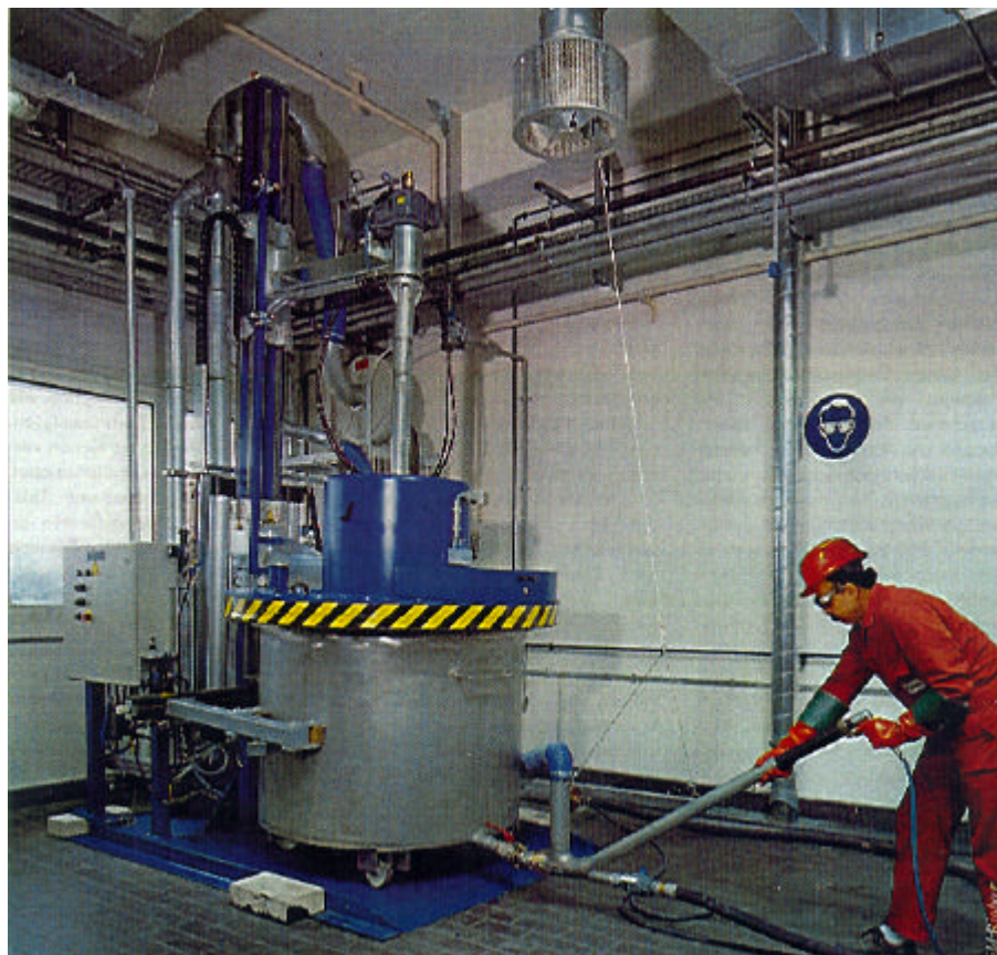
Photo 16: Equipment for cleaning of mobile bin (Riobeer).
