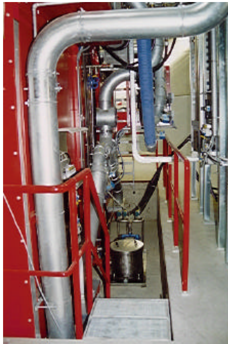
Photo 7: View of rear with runback unit and drying air unit, (Riobeer, IBC cleaning plant CW-III-ex 3D).
