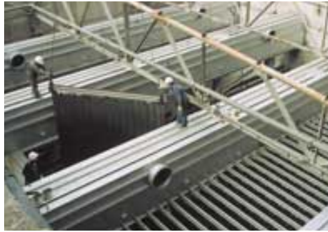
Electrostatic precipitators are being replaced at the Dolna Odra Power Plant, Poland, to reduce fly ash emissions.
