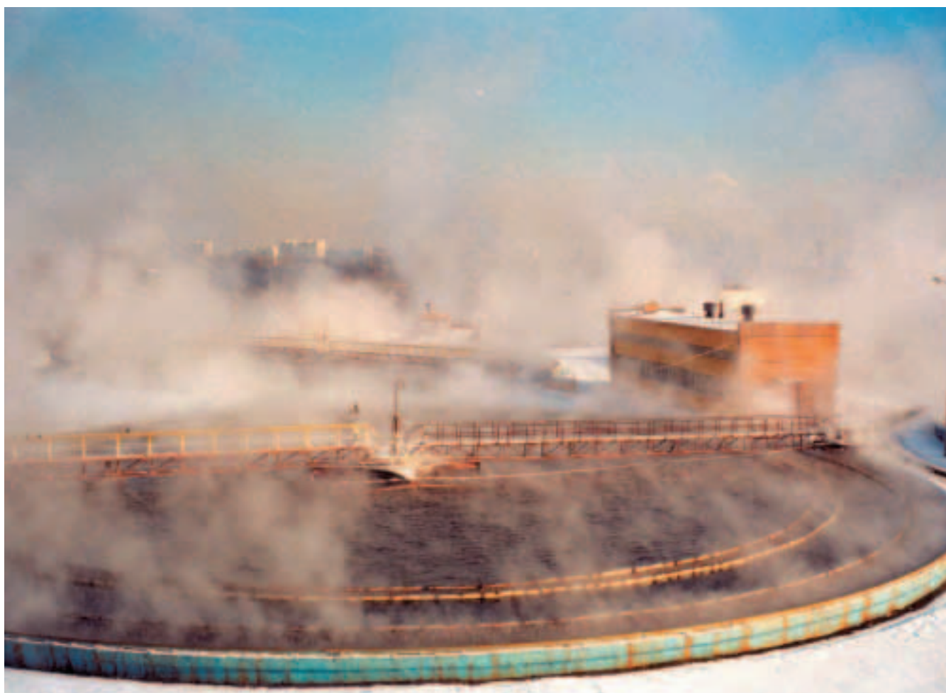
The clarifiers at the Kuryanovo (Moscow) wastewater treatment plant in winter
