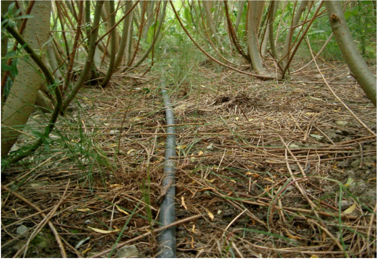
An irrigation pipe lateral placed in a double-row of a willow plantation. (Photo: Stig Larsson)
