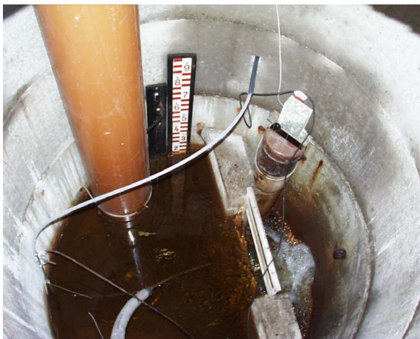
Photo 3.2. Sampling wheel for drain station in the Odderbæk catchment with two stage recorders, V-notched weir and contact switch installed.
