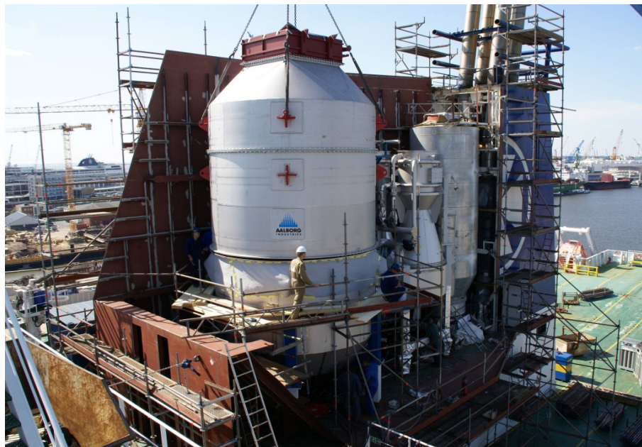
Figure 4-1 Installation of the scrubber system on Ficaria Seawayas (Tor Ficaria) in 2009.
