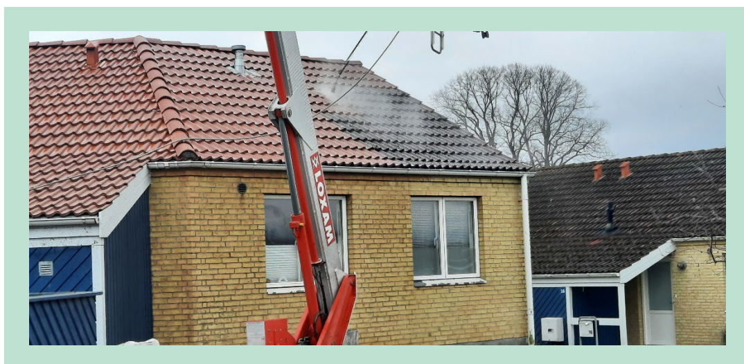
FIGURE 9.9 Professional cleaning a roof in a building complex (use of biocides during this individual operation is unknown).
