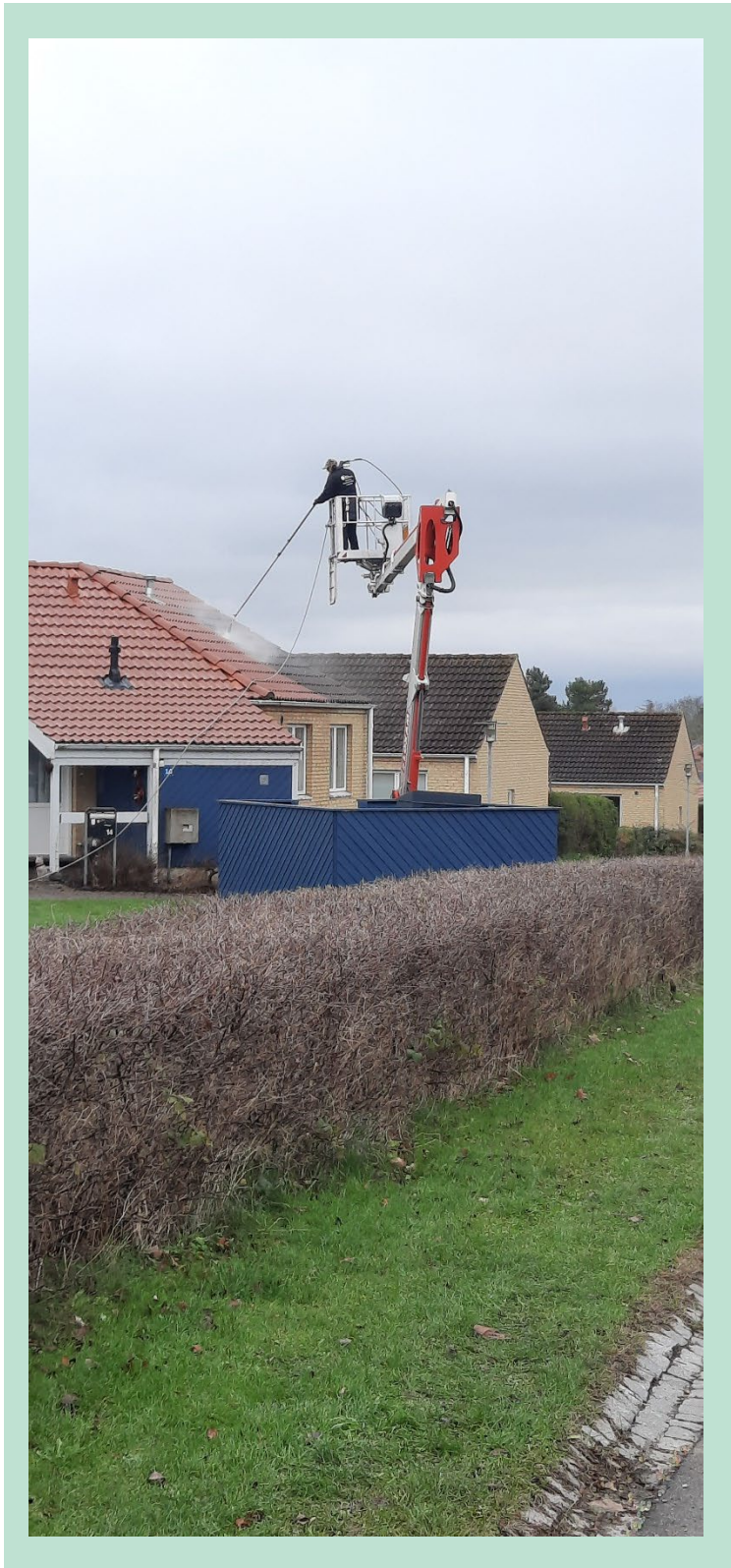
FIGURE 7.9. Professionals cleaning roofs of a building complex (It is unknown which biocides were used during this individual operation).
