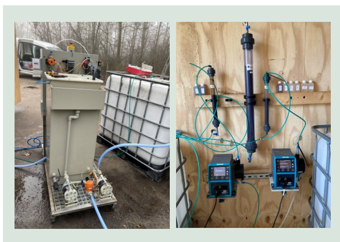
FIGURE 28. Left: Filtration system for treatment after coagulation/flocculation. Right: GAC (the column in the center) and resin columns.
