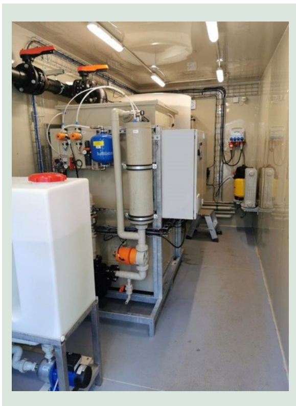
FIGURE 15. Pilot scale test facility at a site in Norway.
